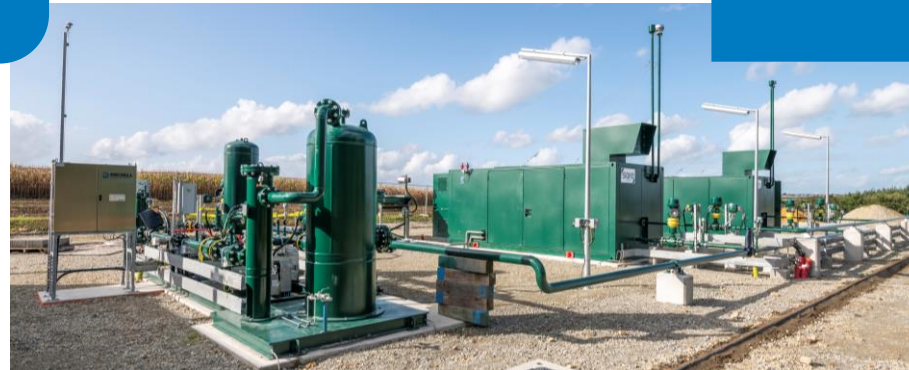
Rebours de Noyal-Pontivy Source GRTgaz
